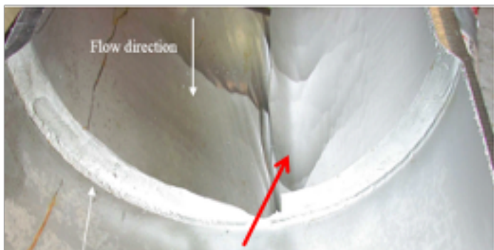
Erosion of internal wall by sand
