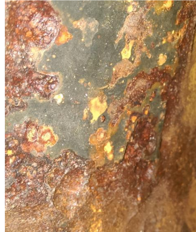
Severe internal corrosion
