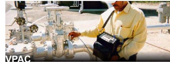
Intrinsically safe valve leak detection loss control
