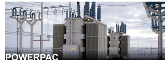
Detecting, locating and assessing electrical & thermal faults in power transformers
