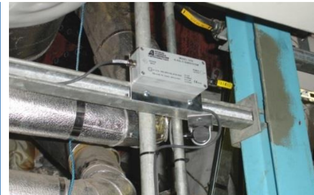
Valve and airborne leak detection
