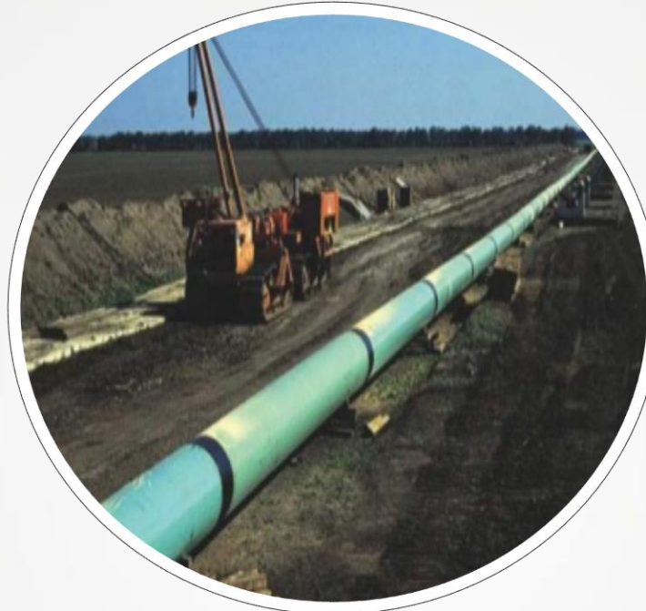
Pipeline (Parallel to ground)
