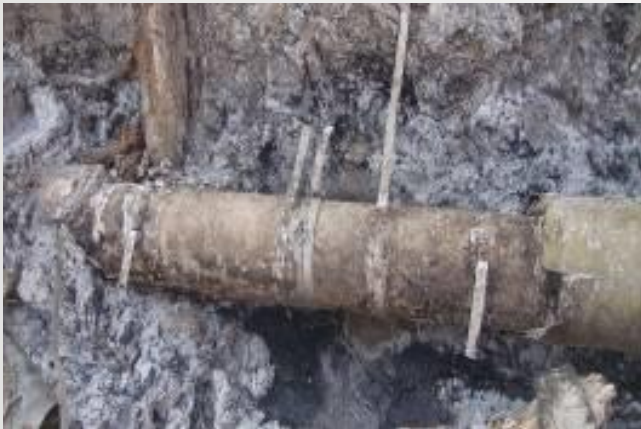
Gathering Pipe Corrosion Perforation
