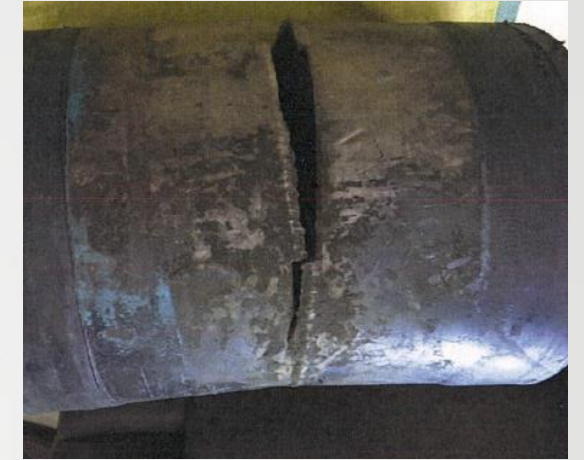
Pipeline Weld SCC
