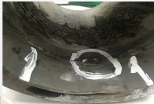
焊缝腐蚀 Weld Joint Corrosion
