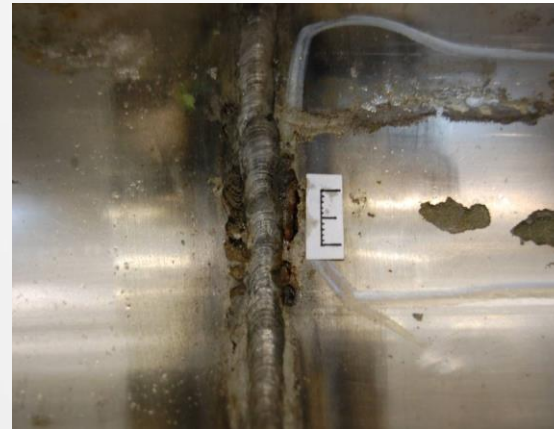
Clad Pipe Weld Corrosion
