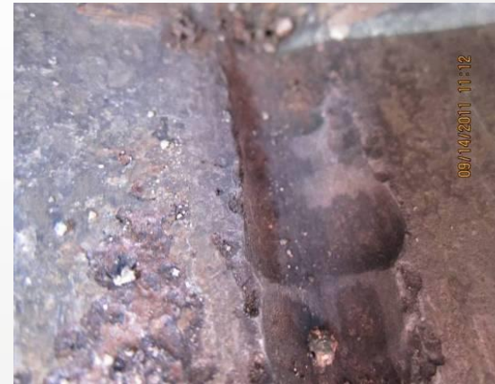
Gathering Pipe Erosion-Corrosion
