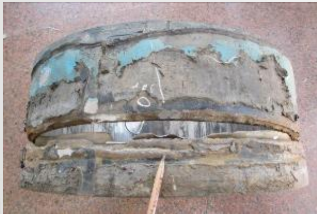
焊缝开裂 Weld Joint Cracking
