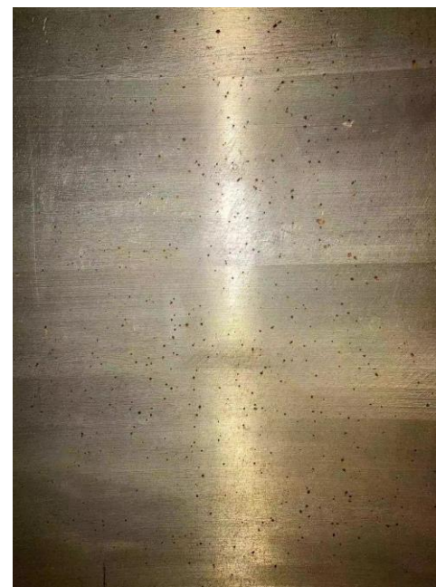
Pitting corrosion of 30408 stainless steel in a domestic organic amine capture system
