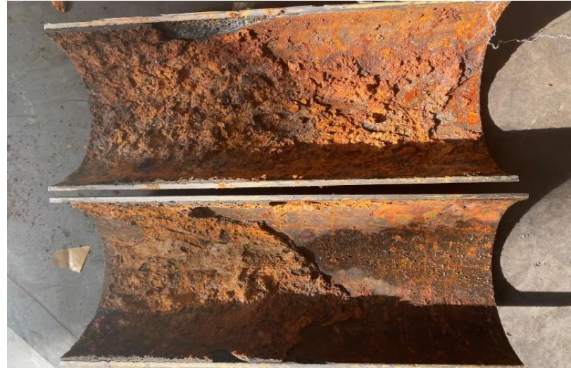
Scaling on the inner wall of production wells
