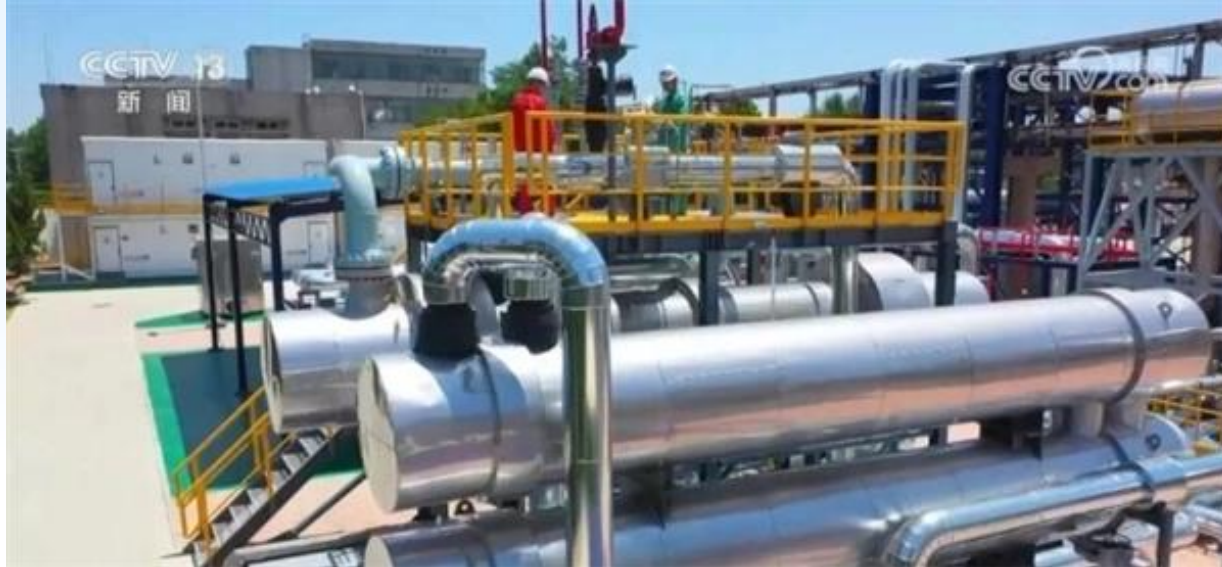
China CO 2 pipeline facility
