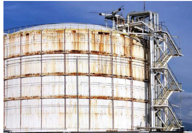
Crude oil storage tanks
