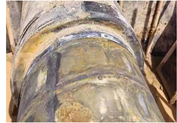
Corrosion under insulation
